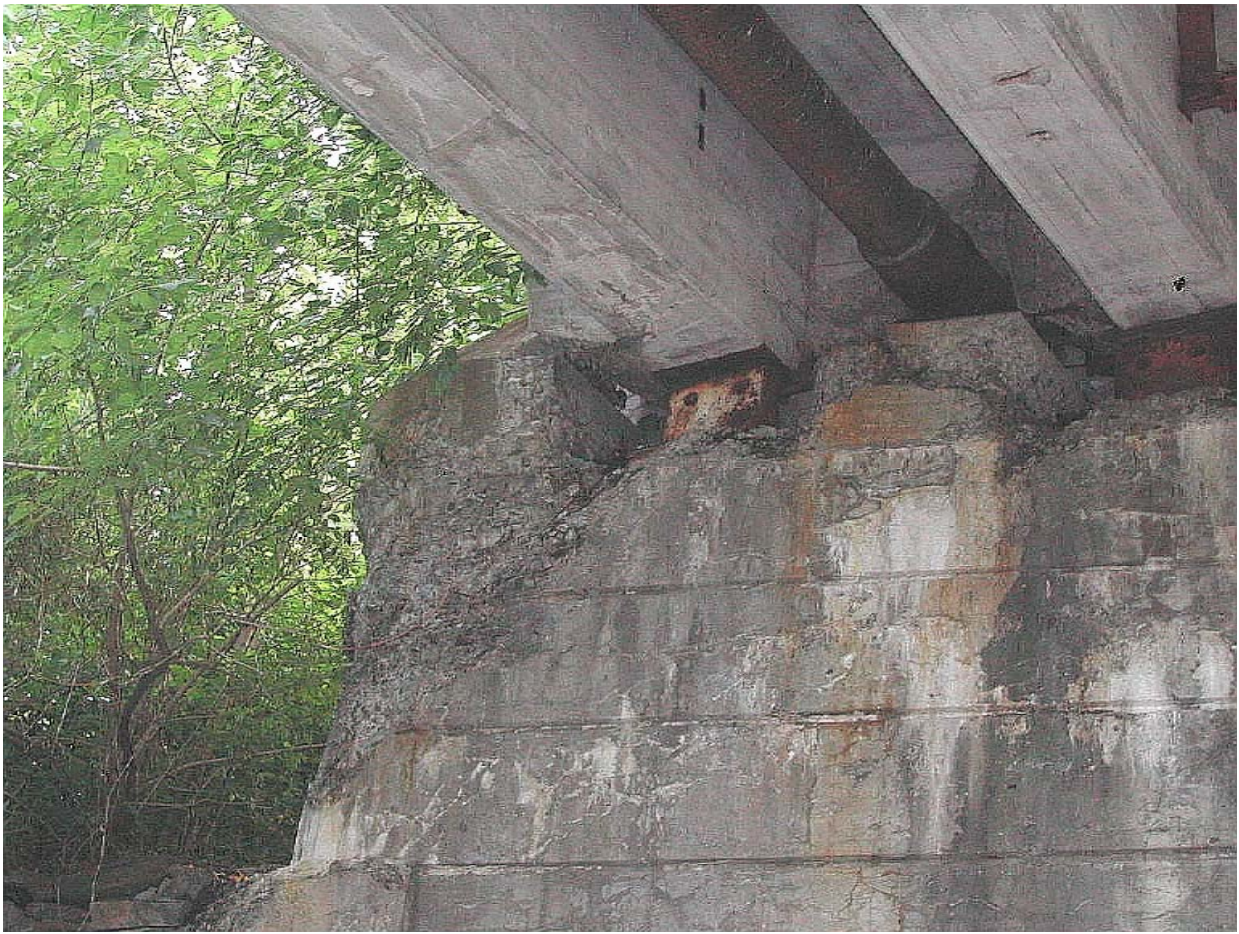
Deteriorating Pier Cap
