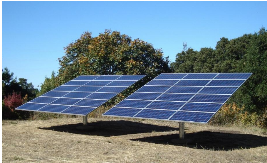
A 5 kilowatt PV system, on two pole-mounted arrays.
