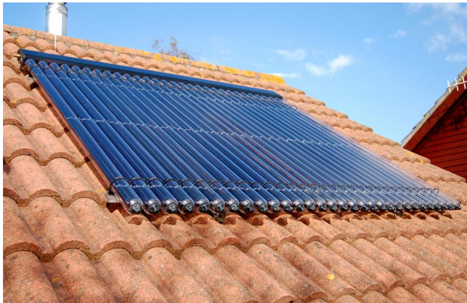
A typical flush-mounted “evacuated tube collector”.
