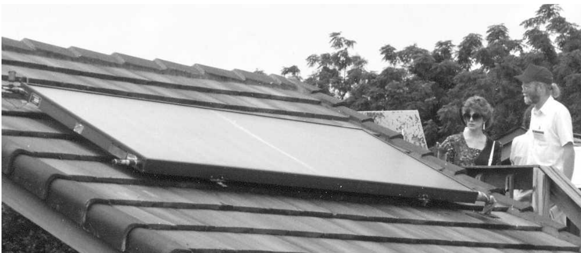
A typical flush-mounted “flat plate collector”.
